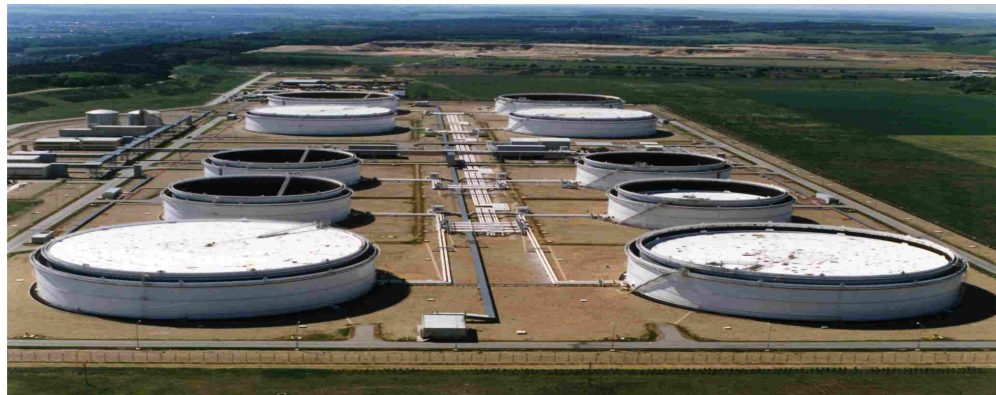
Large-capacity oil tank farm
